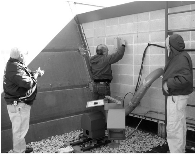
Here Mark Potash (KC9GST) attaches one of the antennas mounting brackets he fabricated to the firehouse wall while Gabe Chido (WI9GC) and Tom Oehler (W9LNL) supervise.
